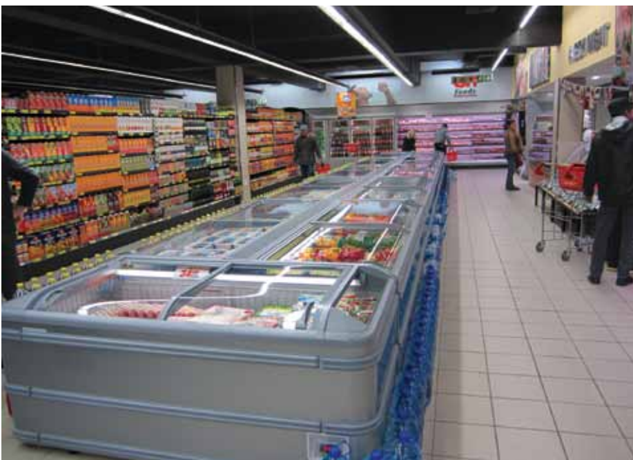
All the old refrigeration was replaced with new-generation closed-waterloop self-contained cabinets. LED lights were used and the fridges and freezers are clean with no ice build-up.
